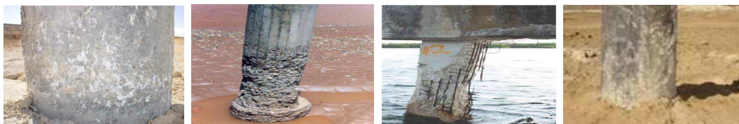
Figure 1 concrete pile damage
