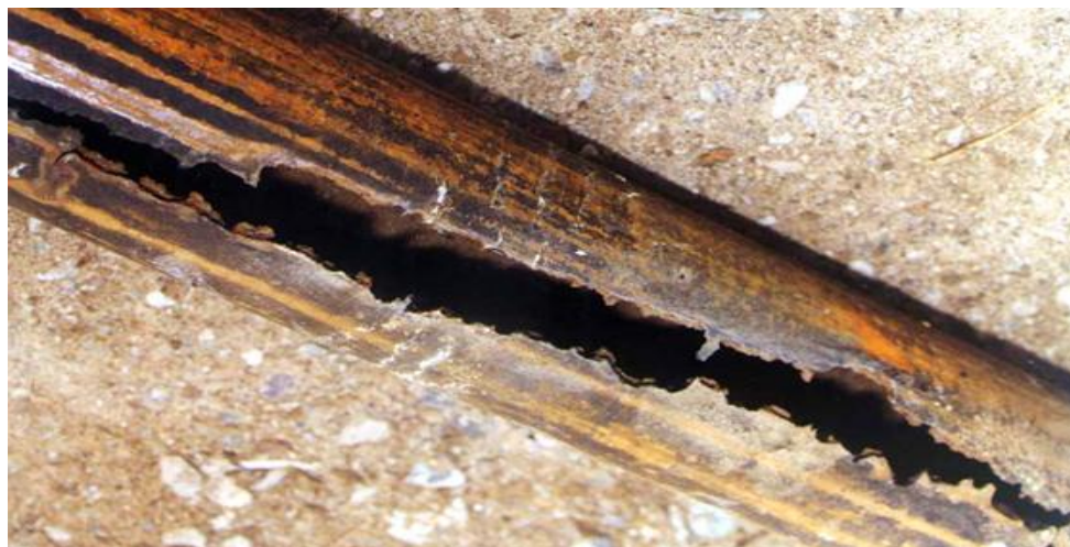
Fig.1: Producing system corrosion of natural gas well under adverse corrosion environments
