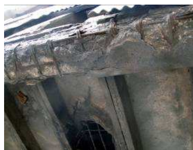
Fig 3: Concrete crumbling and steel bar rusting
