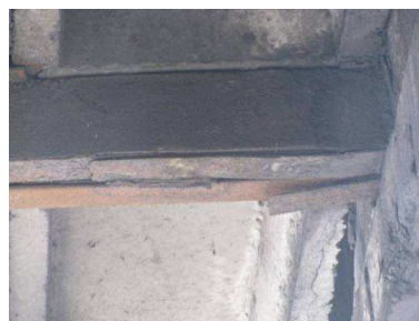
Fig 5: Steel component corrosion serious
