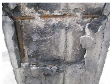
Fig 2: Concrete crumbling and steel bar rusting
