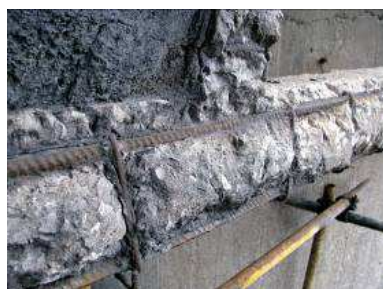
Fig 4: Truss component corrosion serious
